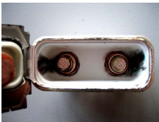
Movable contact / clear signs of arcing
